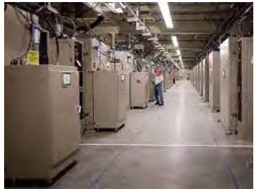
Capacitor banks (~400 MJ)
